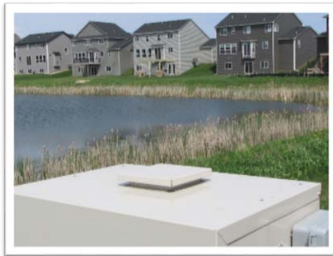
Figure 6. Stormwater irrigation system for residential landscape irrigation in city of Carver, Carver County. Homeowners’ association will manage system.
